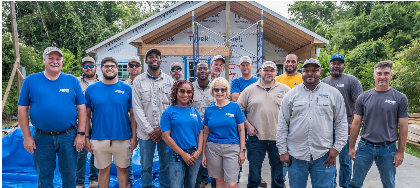
Atmos Energy partnered with Lafayette Habitat for Humanity to build the first ZNE home in Louisiana. Nearly 50 employees volunteered on multiple days to help build the 1,171-square-foot home, which was dedicated to the homeowner in the fall of 2023.
